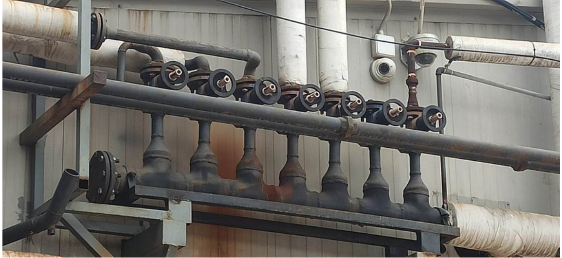
Image 8: return loop manifold
