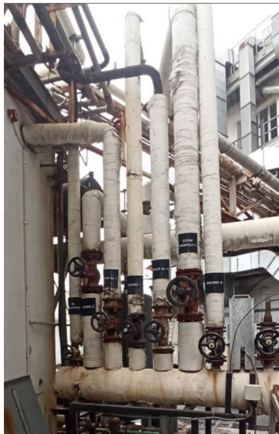
Image 7: Steam distribution manifold
