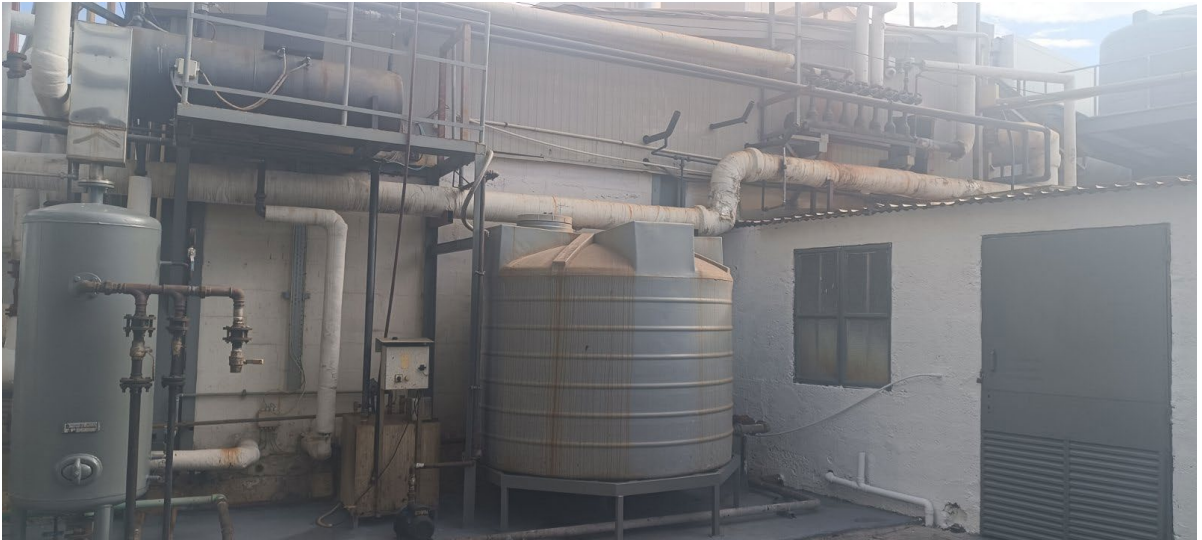
Image 6: Feed water tank
