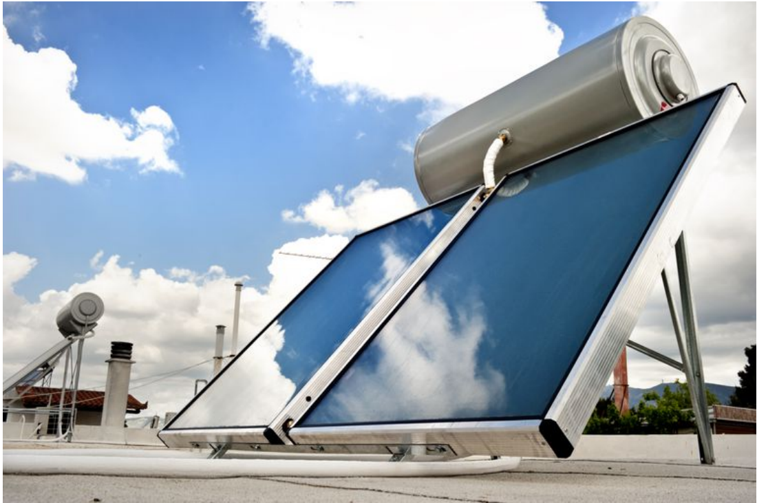
Picture 20: Solar water heating (West, 2020)
