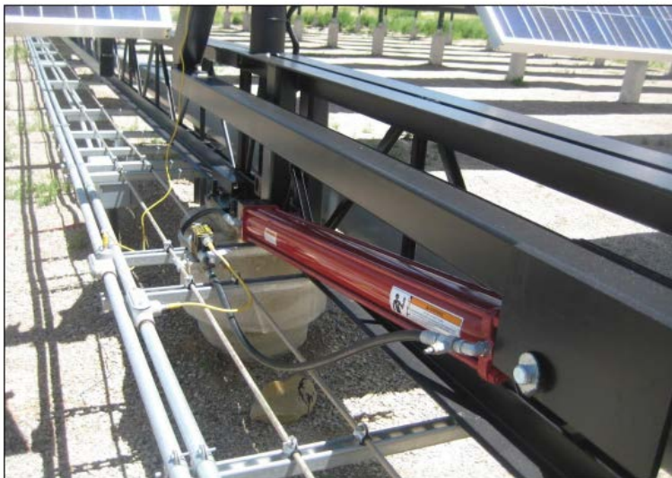
Figure 15. PV Modules With Tracking System (Pearsal, 2016)
