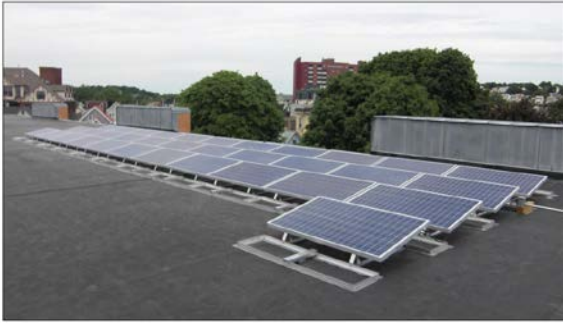
Figure 12. PV rooftop installation (FAA, 2018)
