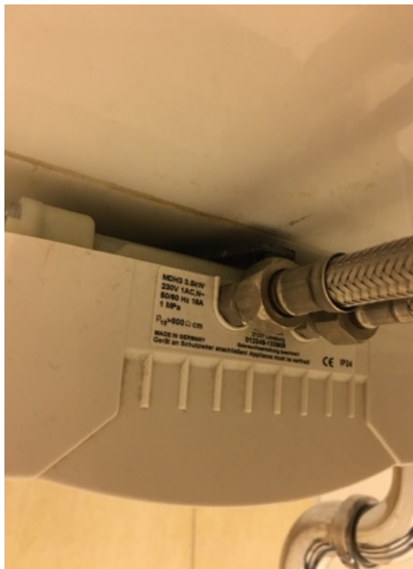
C.5: Electric Water heaters used by the company
