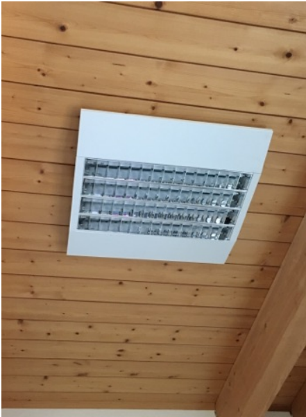
C.1: Fluorescent lamp
