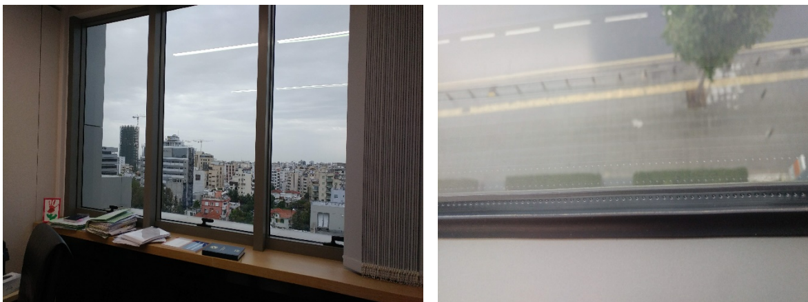
Photo 8 Reclining windows of the sixth floor and a view of the inside of the window
