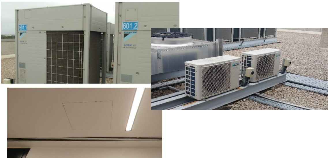
Photo 10 Outdoor VRV and Split Units. Air- conditioning and ventilation louvers of the concealed indoor units
