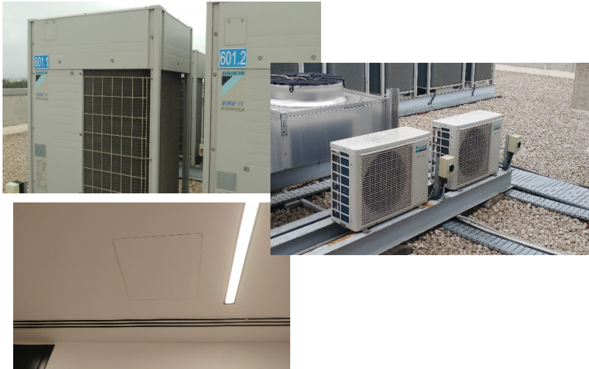
Figure 3. Photos of the installed variable refrigerant flow units and air conditioning on the rooftop
