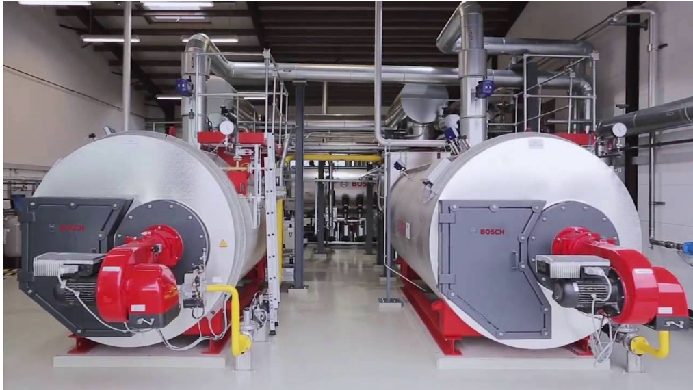
Picture 20 Steam Boiler (Bosch, 2023)
