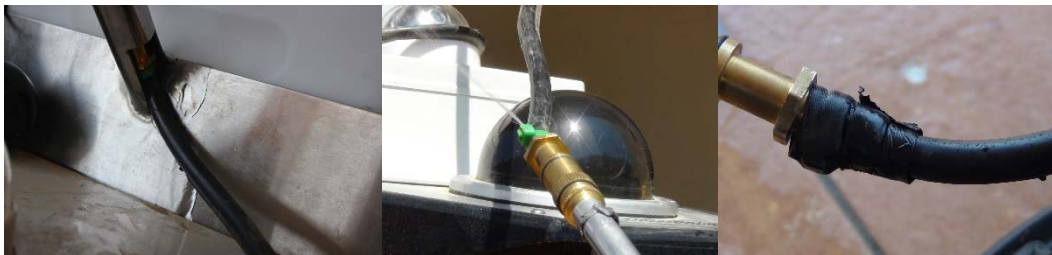
Figure 11. Fractured hose problem - Left: friction caused the problem, Center: the actual problem water leakage, Right: problem fixed with reinforced binding tape
